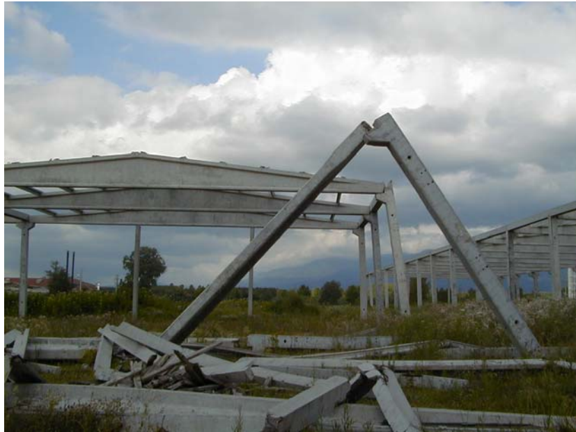
Figure 1.8 Photograph of a Completely Collapsed Precast Building
